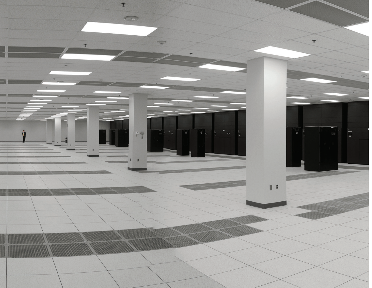
Shell managed wholesale raised floor, image courtesy of QTS
