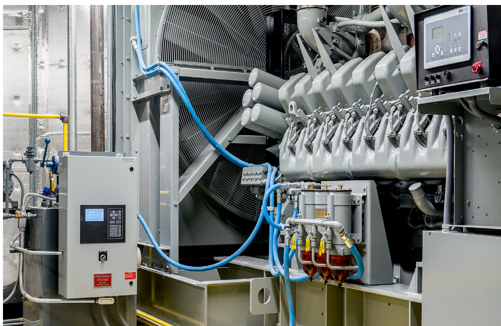
Figure 13-Diesel generator, image courtesy of ViaWest
