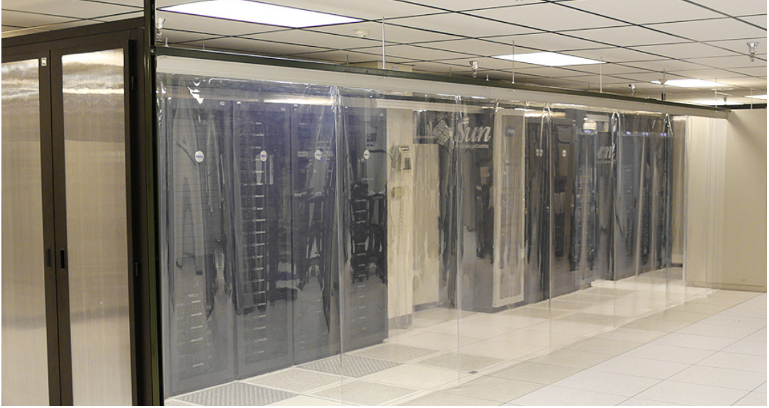
Figure 25-Photograph of hot and cold aisle containment
