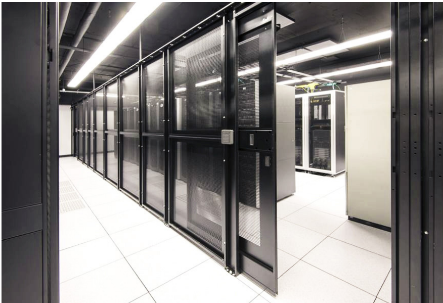
Private cage on raised floor, image courtesy of Cologix
